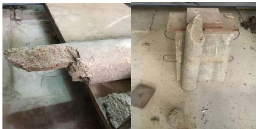
Fig.6: The failure of piles reinforced with carbon fibre bristles.
